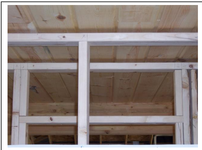
Figure 16. Interior walls showing the gap between the wall and the ceiling.
