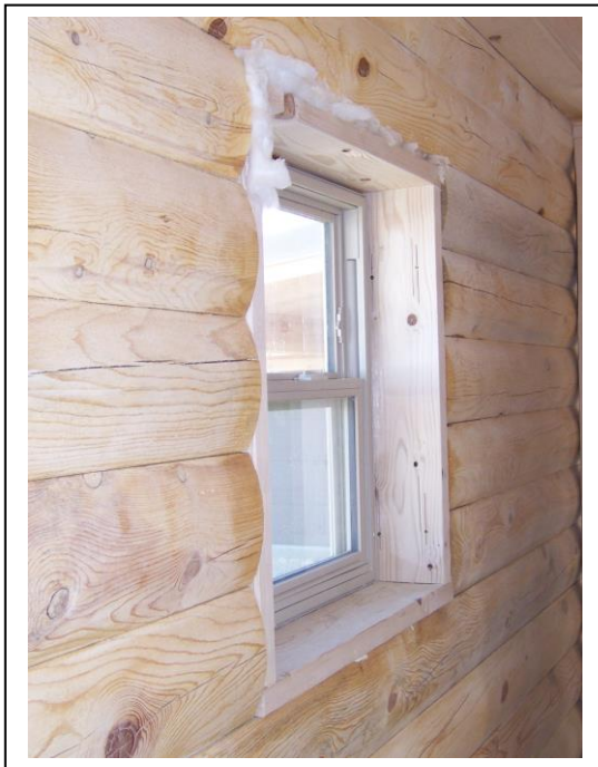
Figure 11. Window buck and window that have been secured in the window opening.
