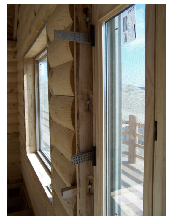
Figure 13. Inside view of the door buck and door mounted in the door opening.
